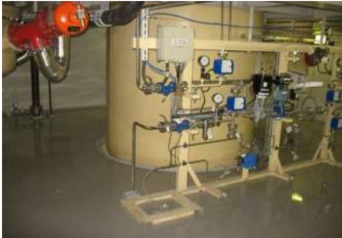
Combustible solid RW incineration facility with gas purification
